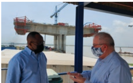
NSIA Managing Director and Chief Executive Officer, Mr. Uche Orji, in discussion with the site engineers at the Second Niger Bridge.
