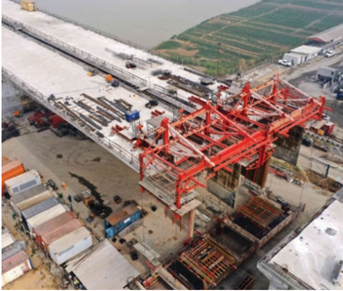
The Second Niger Bridge under construction – Catalytic, high priority infrastructure is a priority for the Board.
